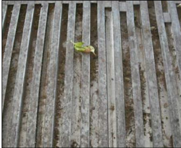
Soil contamination on a container floor.
